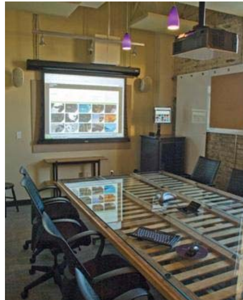
Presentation-capable conference rooms have access to a VBrick video hub that stores and distributes video throughout the office space.
